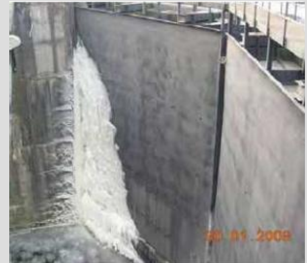
Ice occurrence in locks on the Danube preventing their operation. Source: via donau.
